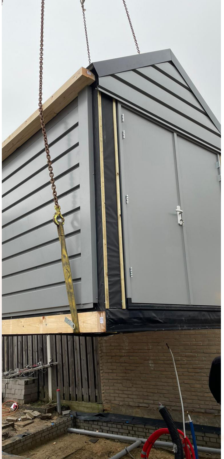
Installation of a prefabricated module with heat harvesting walls, roof and equipped with a heat pump
